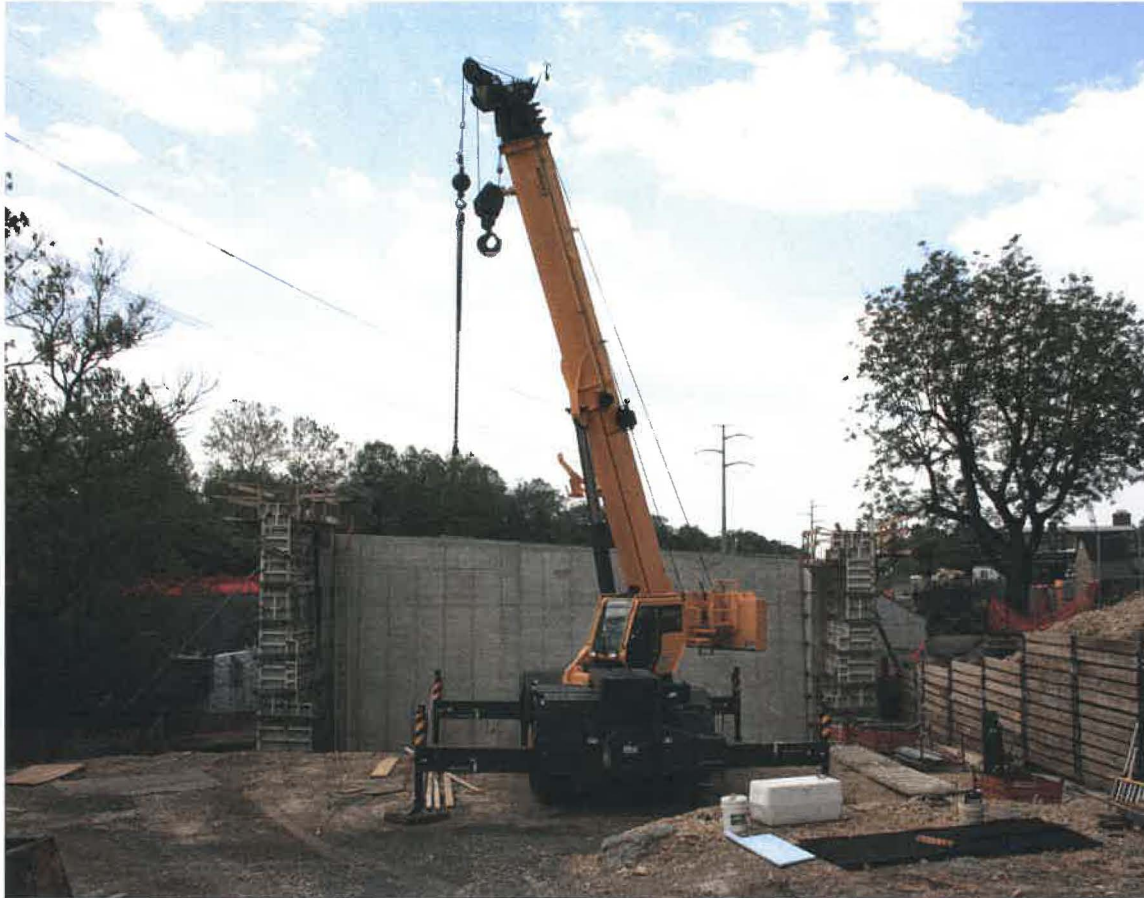
The Lafayette Street extension in Norristown and Plymouth leads to a project listed as a Vision Roadway Project, the Lafayette/Ridge interchange of I-276, the Pennsylvania Turnpike.
