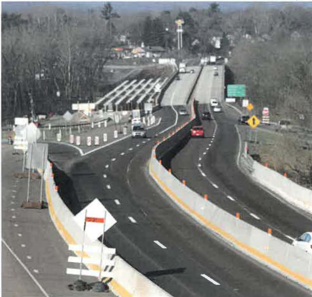
The reconstruction of Route 422 over the Schuylkill River was listed as a Transportation Improvement Program project before being let for construction.
