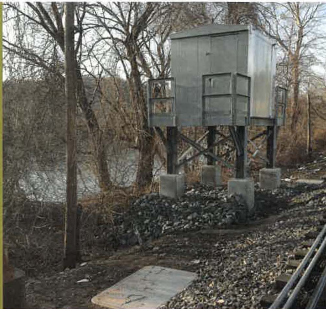
This elevated train signal hut illustrates changes designed to make infrastructure more resilient to flooding and climate change.
