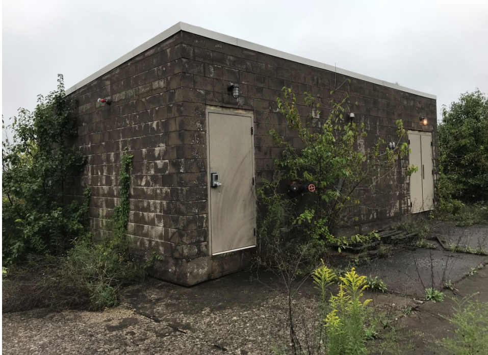
Photograph 15. Firefighting Pump House
