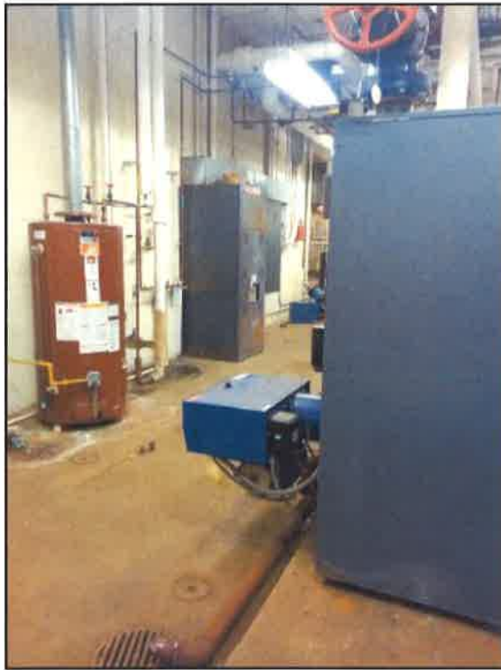
Photograph 11: Floor drains observed in boiler room of administration building.
