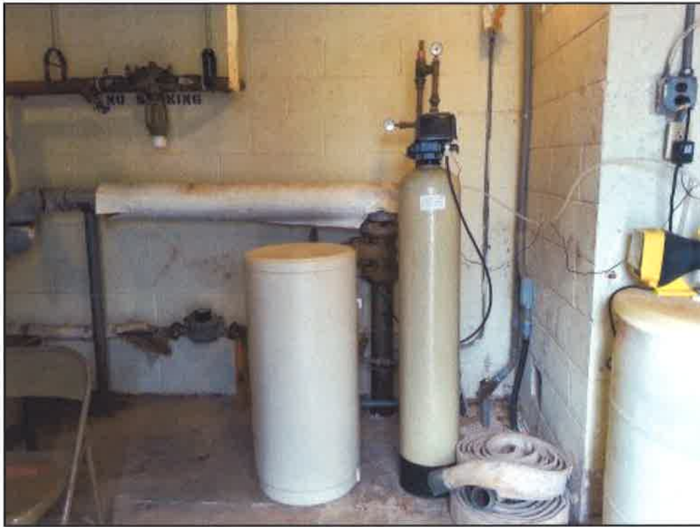
Photograph 15: Potable water treatment system.
