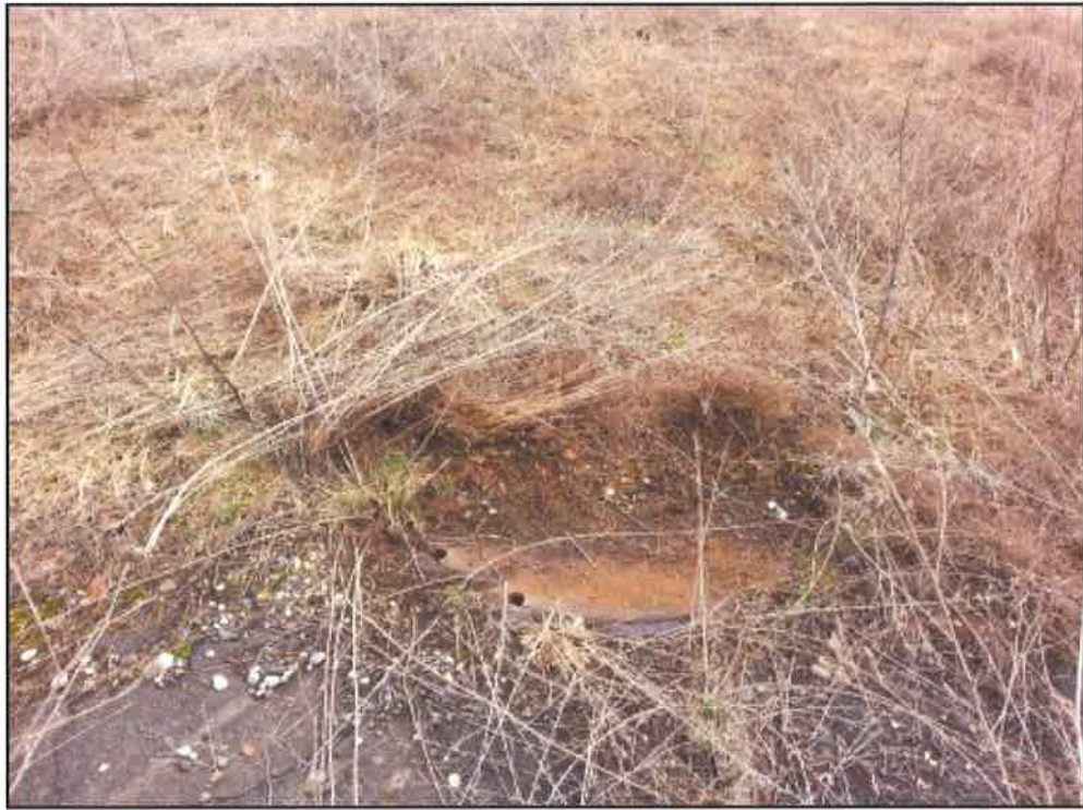
Photograph 31: Manhole cover located in bermed area.
