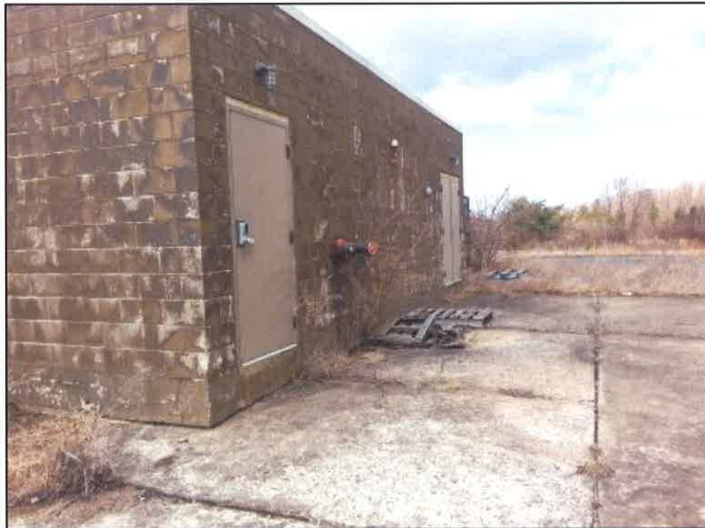
Photograph 26: Fire protection pump house located on top of center missile silo.
