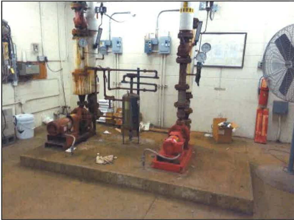
Photograph 5: Two pumps located in boiler room of administration building.
