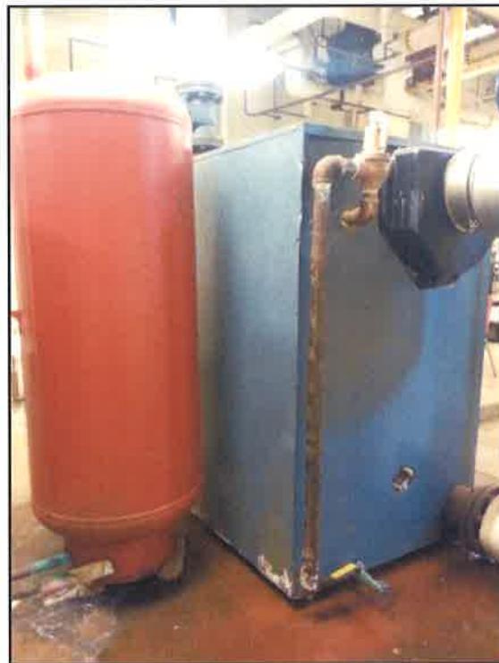
Photograph 10: Boilers with condensation water around their base.
