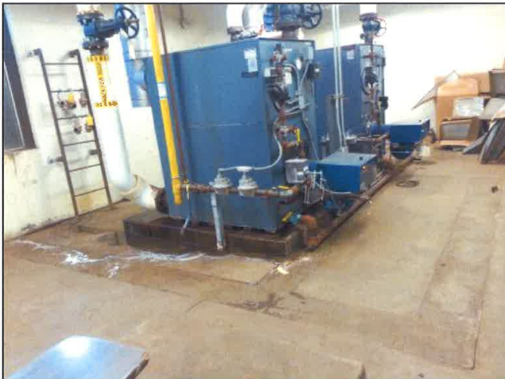
Photograph 6: Boilers located in administration building.
