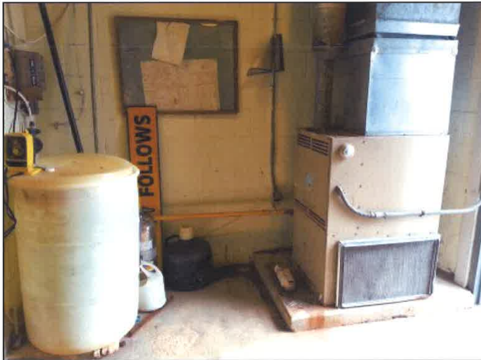
Photograph 16: Heater inside potable well house.
