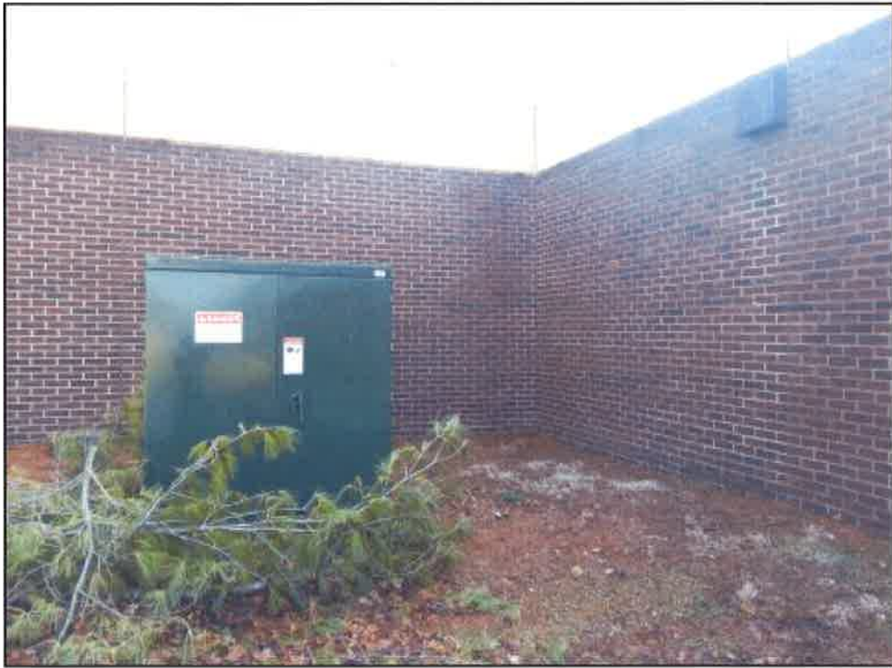
Photograph 27: Pad mounted transformer.
