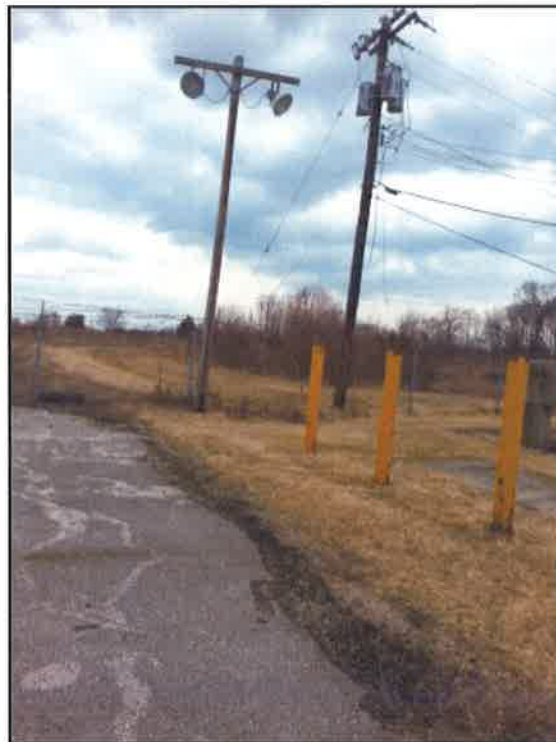
Photograph 28: Pole mounted transformers.
