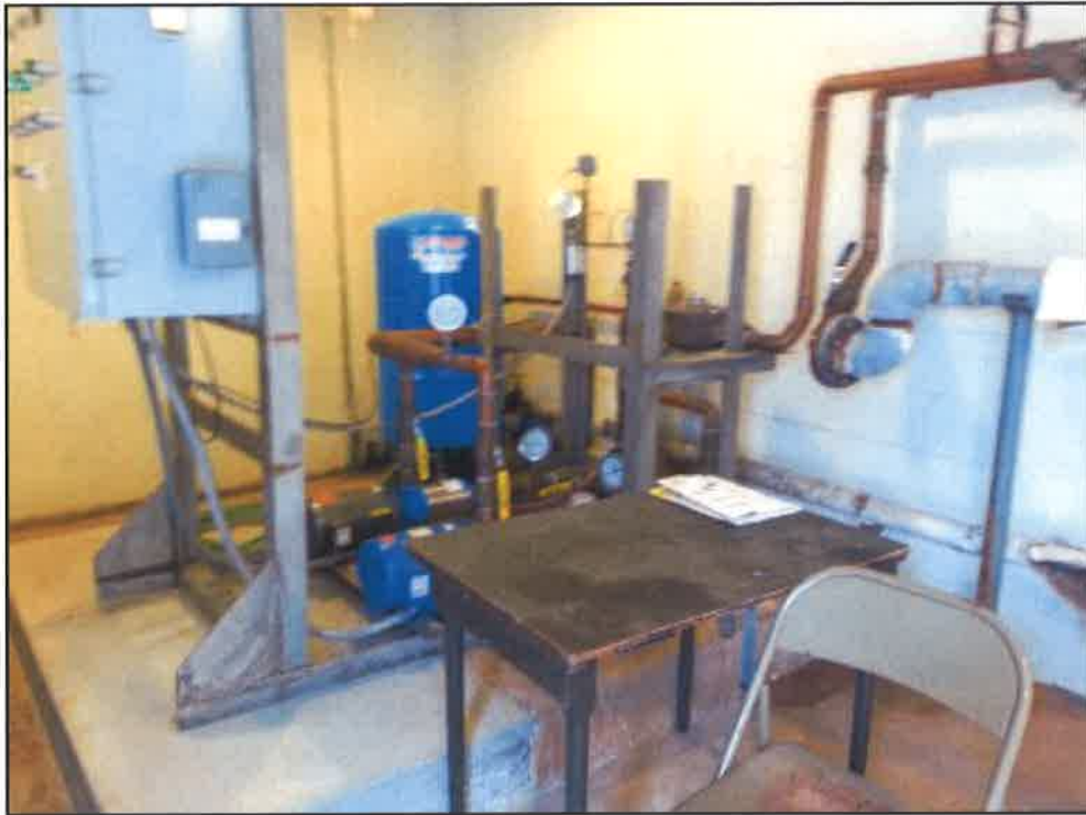
Photograph 17: Pumps located in the potable well house.
