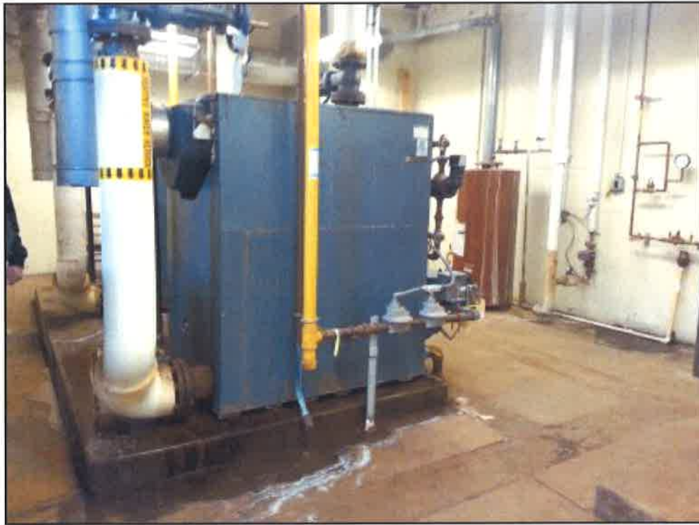
Photograph 9: Boilers with condensation water around their base.
