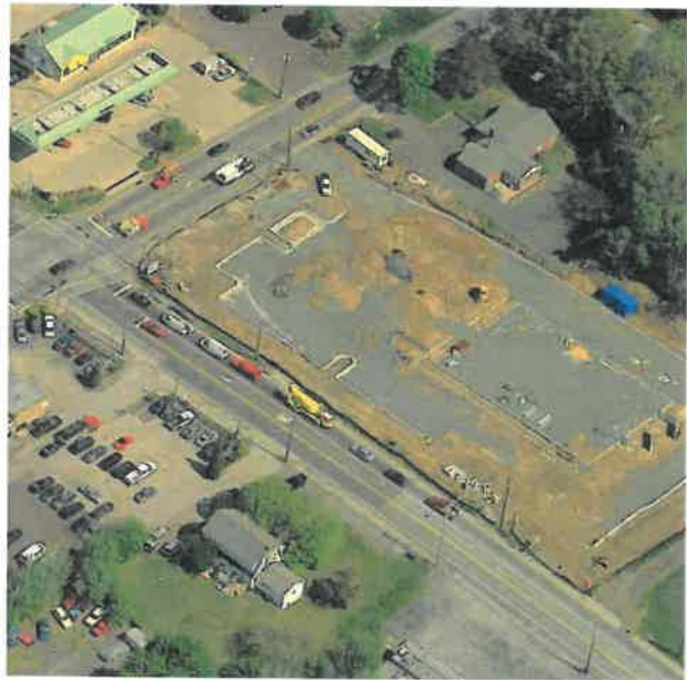
Eckerd drug store construction at Germantown Pike and Valley Forge Road. This was completed in 2005. Pictometry
